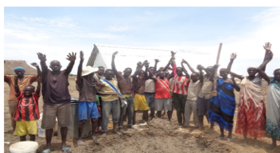
Community members ready for the mudding of the new structure in Nasir.
